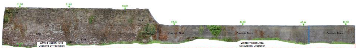
Fig.8: Protected brickwork and concrete walled garden at the southeast of the site, proposed for demolition. Source: Murphy survey
